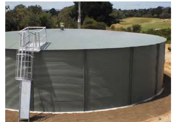
Water Tanks To harness stormwater
