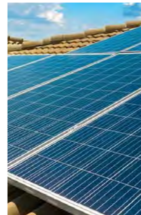
Solar Panels To new buildings
