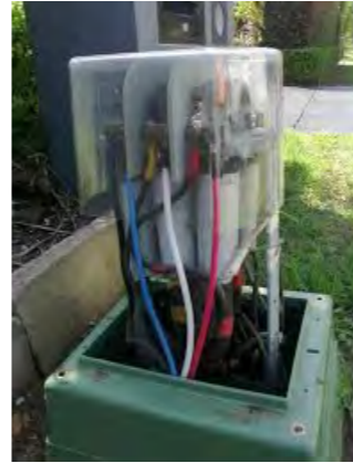
Additional Electrical Points For Events (Henry Street)
