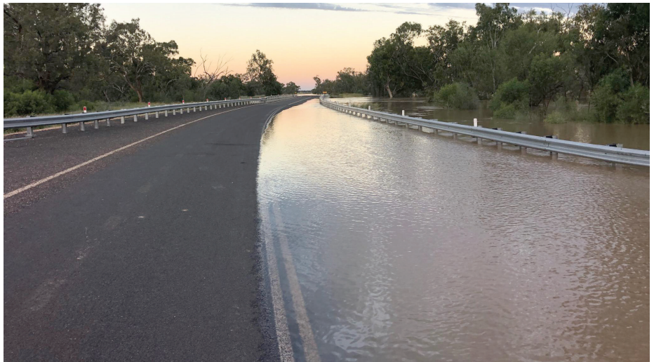
Flood water crossing the Thallon-Noondoo Road at the Thallon Bridge.
