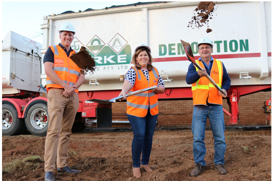
LET'S GO: Mayor Samantha O'Toole and Cr Rod Avery launch construction of the St George Library Hub with St Hilliers Site Manager Ryan Canning.
